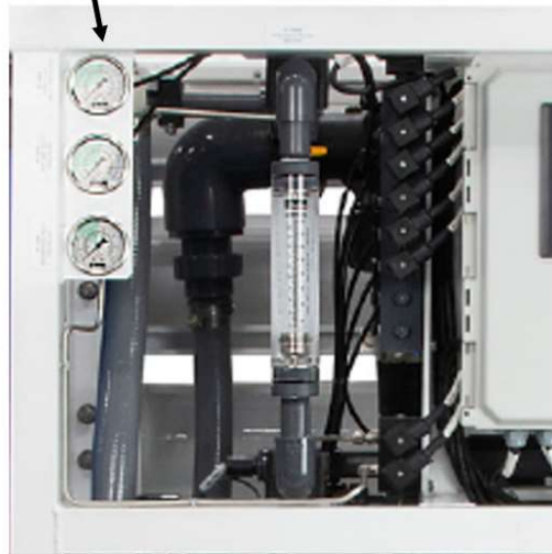
Figure 5.1 – View of Gauges
