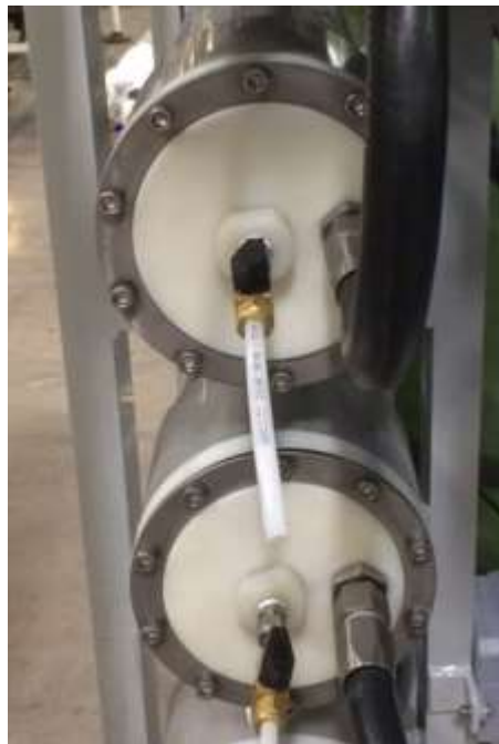
Figure 7.9 – Pressure Vessel Plumbing
